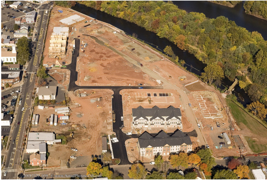
Photo of the site taken in October 2005 showing that the remediation was completed and construction was underway.
